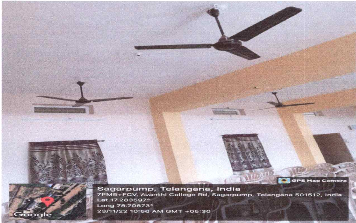
Back-up Energy using to all class Rooms
