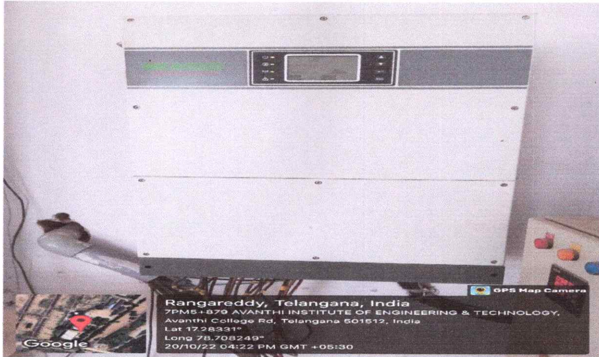
BLOCK-I Solar plant connected to power grid
