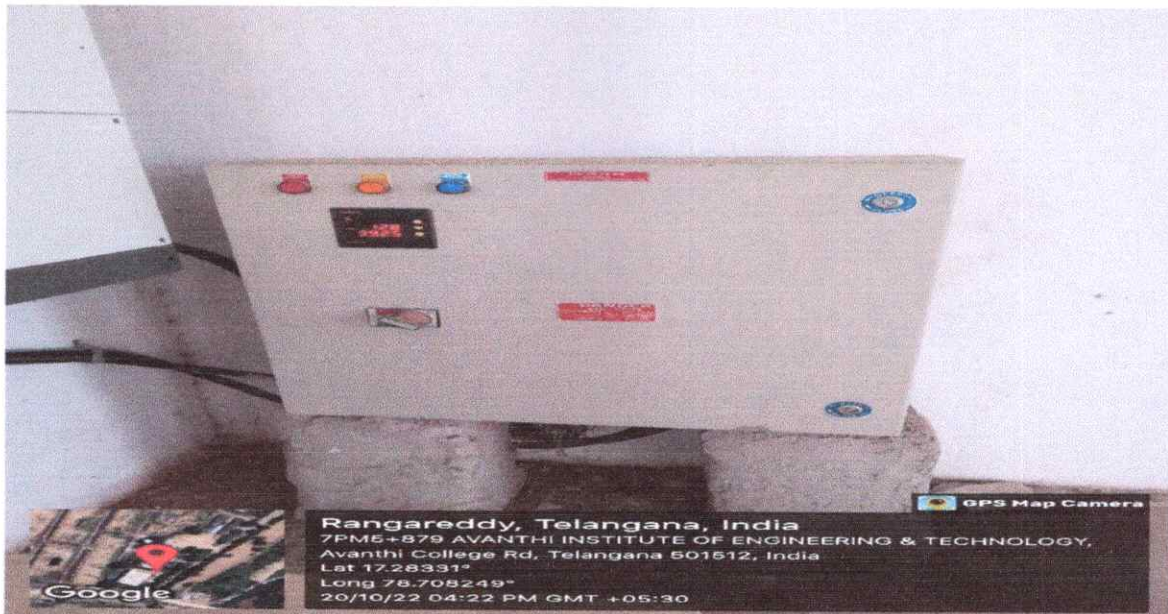
BLOCK-II Solar plant connected to power grid
