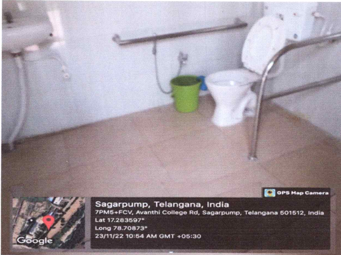
Divyangian-Friendly Washrooms In EEE Block
